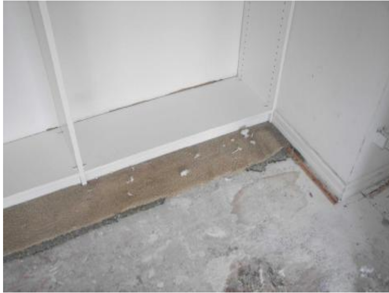
Water damage to upstairs master bedroom flooring and closet organizer
