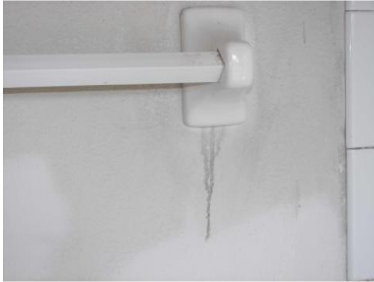
Smoke and water damage to master bathroom
