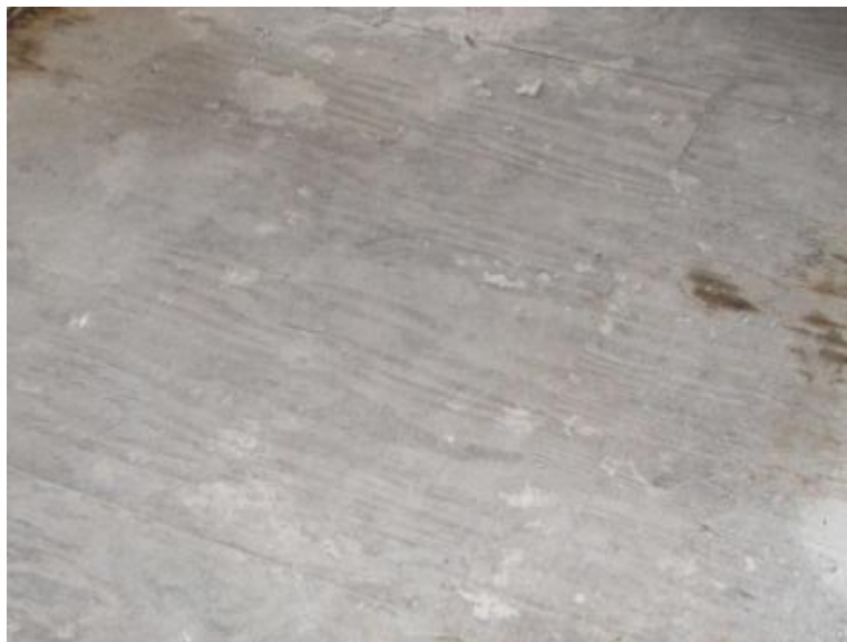
Water damage to upstairs hallway subfloor
