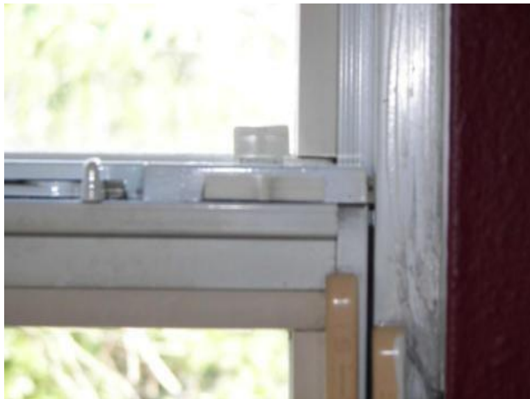
Smoke damage to windows
