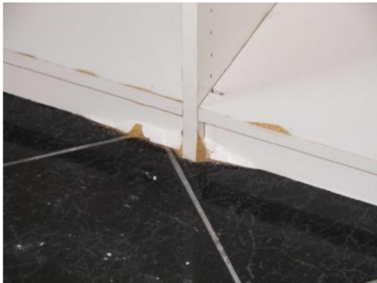
Water damage to upstairs bedroom 4 closet organizer
