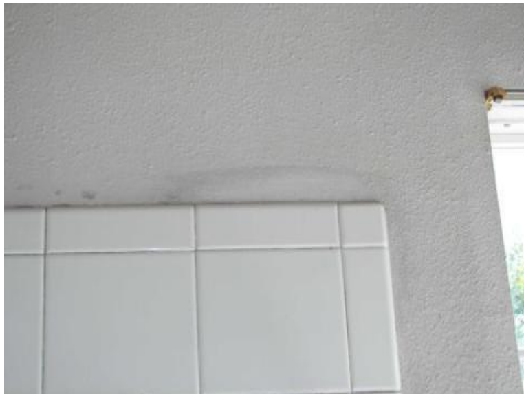
Smoke and water damage to master bathroom
