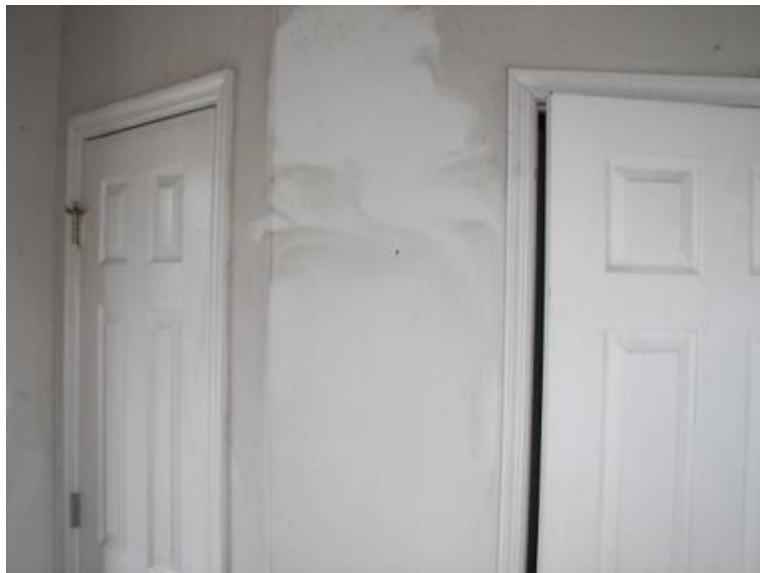
Smoke damage to master bathroom
