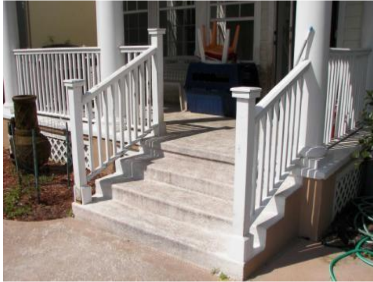
Smoke damage to upstairs porch
