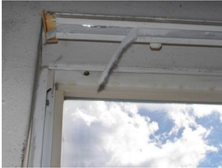
Smoke damage to windows
