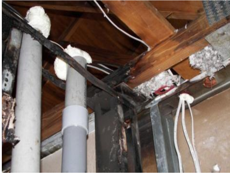
Fire damaged ductwork in the laundry room
